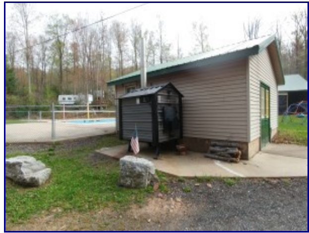
Wood furnace for the pool
