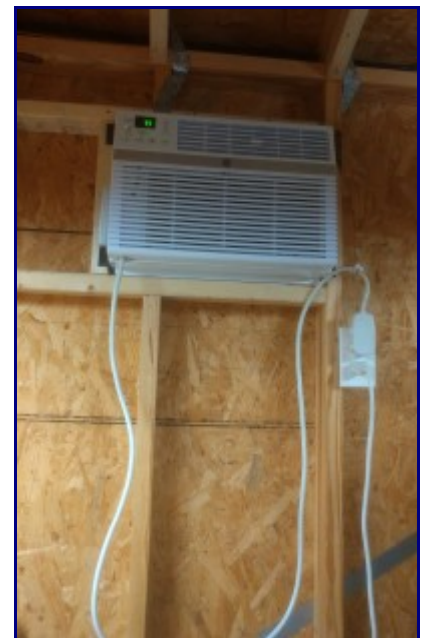
Air conditioner installed
